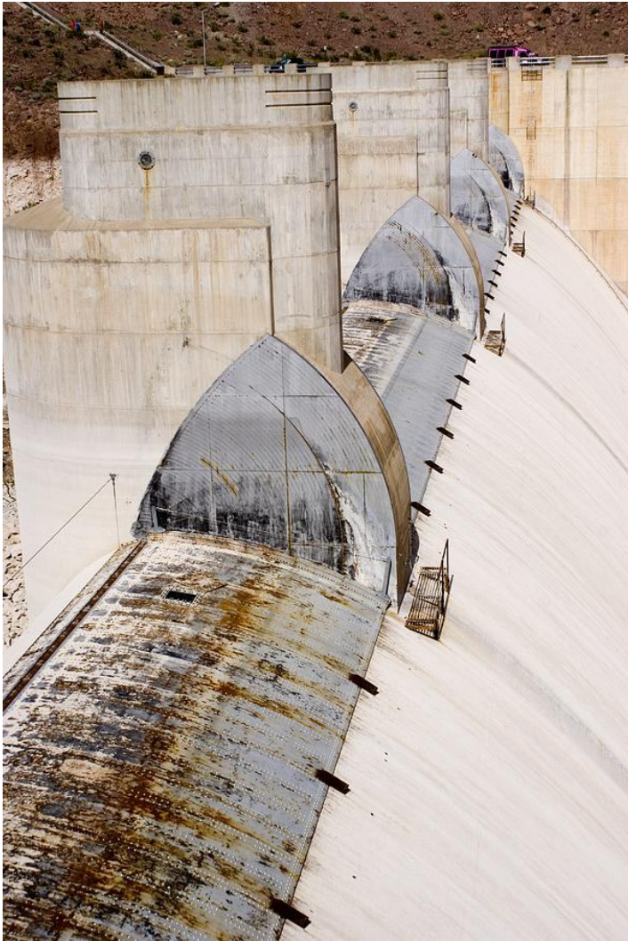
Sluiceways of Hoover Dam now rusting...
